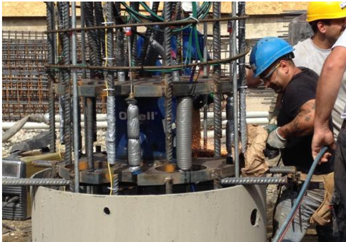
Figure 8. O-Cell and TIP cables
